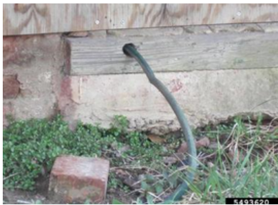
Openings near utilities
