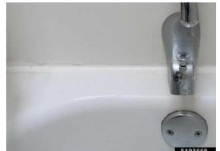
Leaky pipes or faucets
