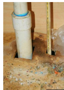
Openings near pipes
